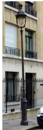
Eclairage public - Luminaire
